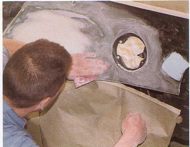
A slight blemish was found, so it was sanded down immediately, as primer-surfacer will be sprayed as soon as masking is completed. With that blemish touched up, masking is finished up by adding masking paper along the bodyline where the rear bumper/fascia abuts, and upward along the back edge of the rear quarter panel.
