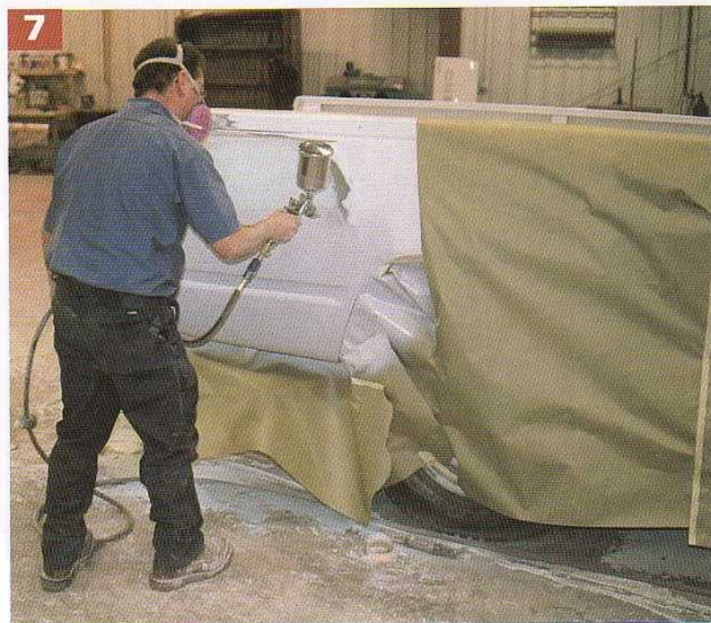
Apply primer-surfacer with each pass extending past the actual repair area slightly and onto the masking paper. In this case, paint will cover the repair from around the back edge to the edge of the wheelwell, so the primer-surfacer must be applied there as well.
