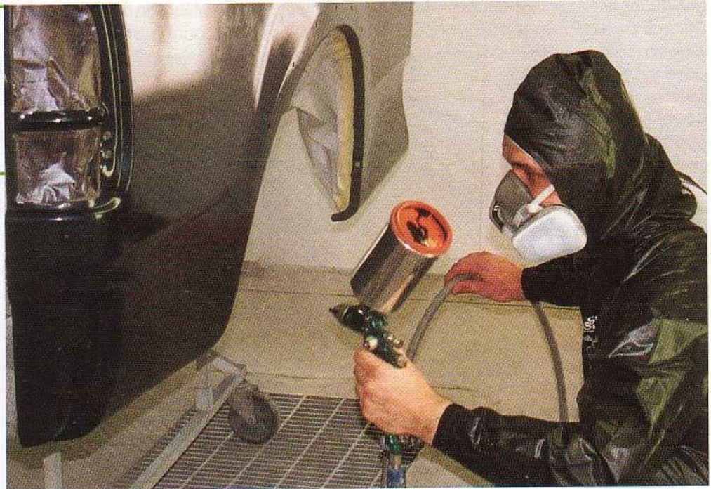
Kneeling helps this painter see where he's applying the clear. Notice how he took the time to mask the inner wheelwell and the inside of the bed of this pickup truck.
