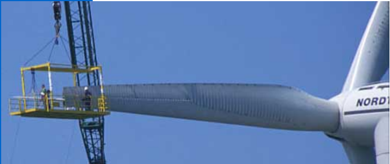
Service crew working on a 32 m rotor blade on a 1.5 MW wind turbine
